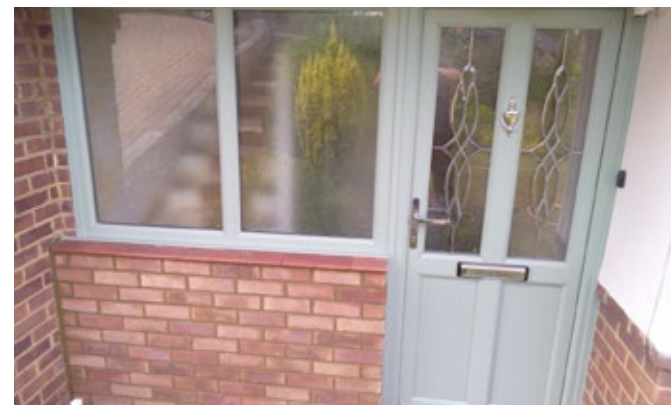
Specialised property flood resilience door, reducing ability of water to enter via the door.
