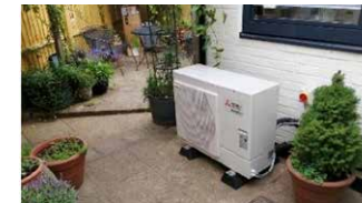
Rear garden – ground mounted
