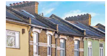
PV installation on several roofs
