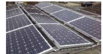
Concertina PV installation
