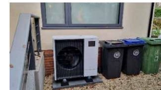
Front garden – ground mounted
