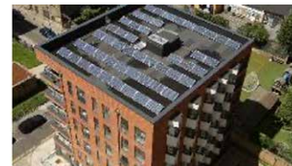
PV installation on building with flats
